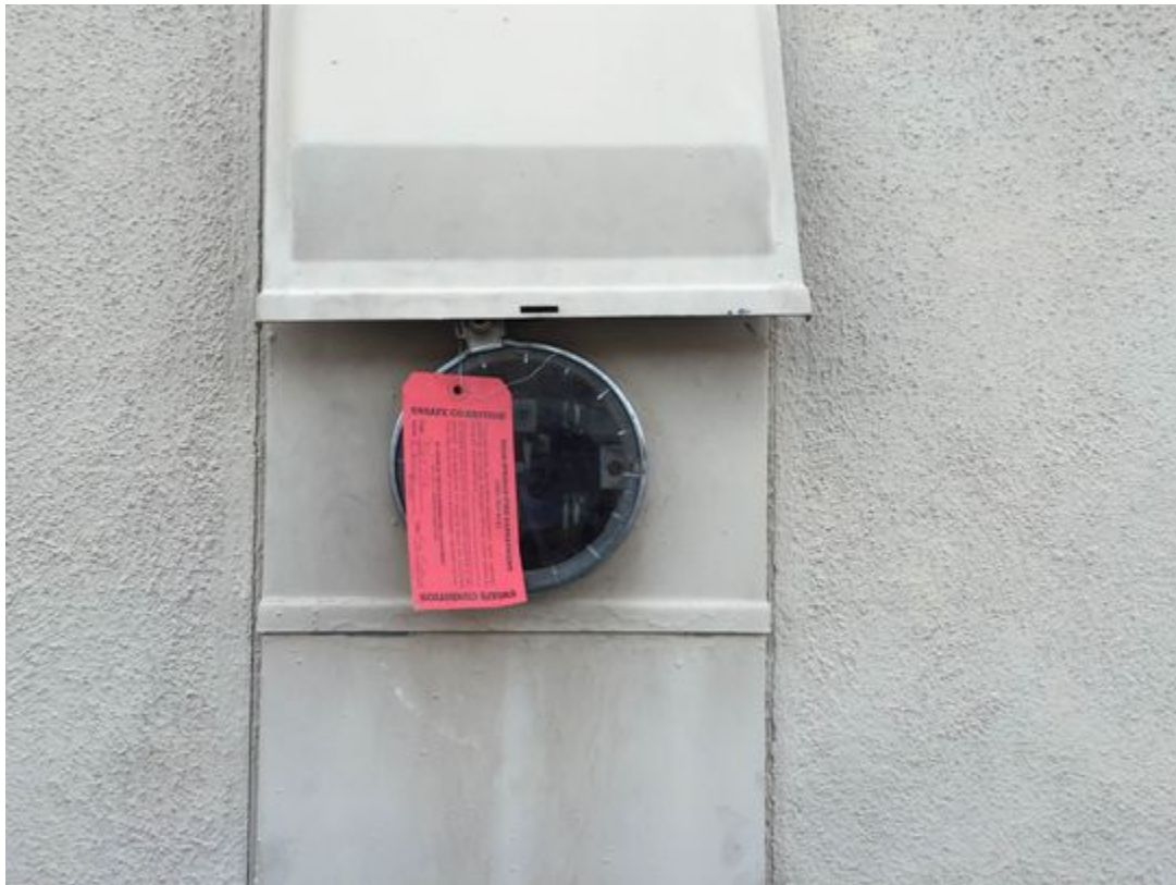
A tag on the electrical meter at a house in Palm Springs identifies it as unsafe after an electric shock in a pool on March 27. (Rosalie Murphy/The Desert Sun)
